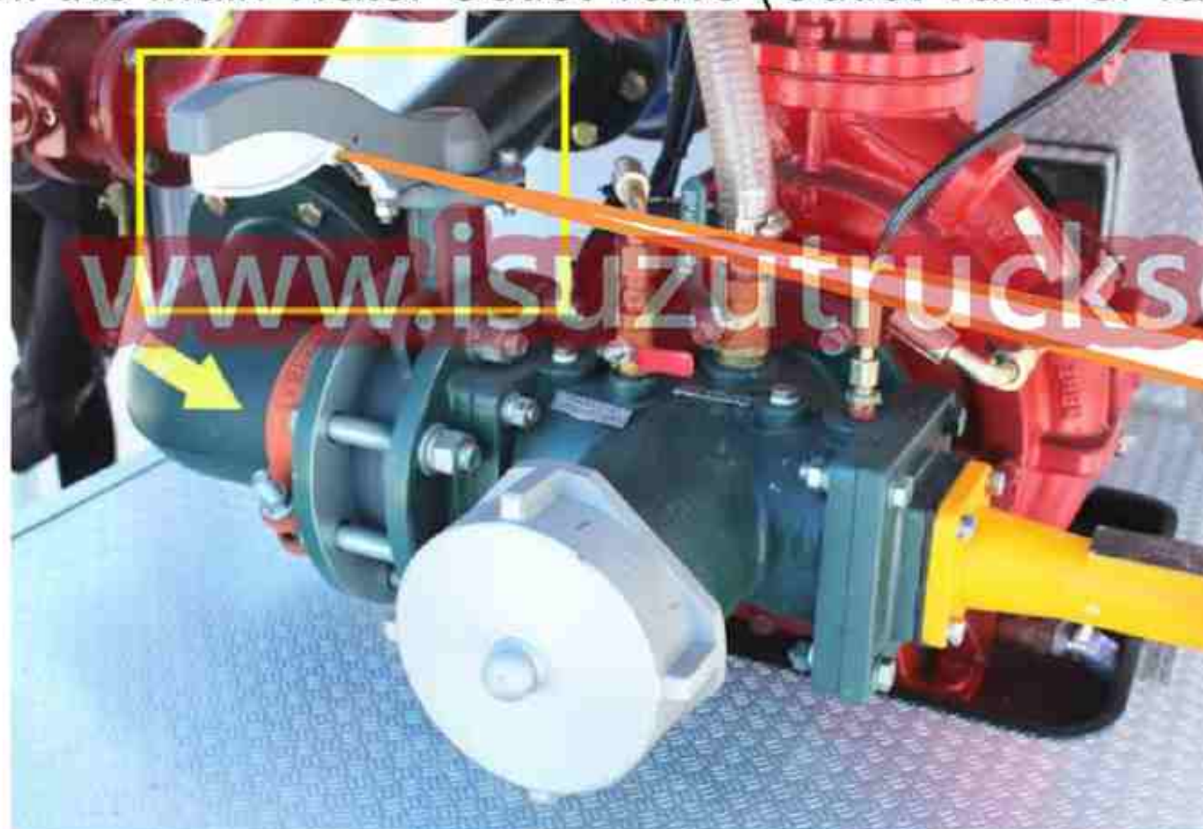
Turn off the Outlet Valve of Tank
